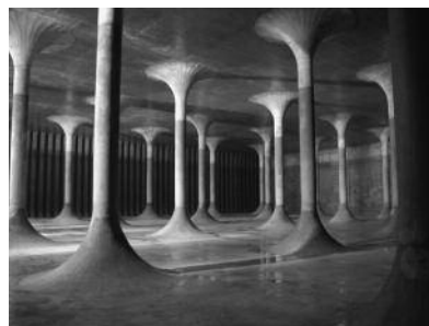
Reinforced concrete pillars in the underground cistern of the Budapest Waterworks on the Gellért Hill from 1980.
