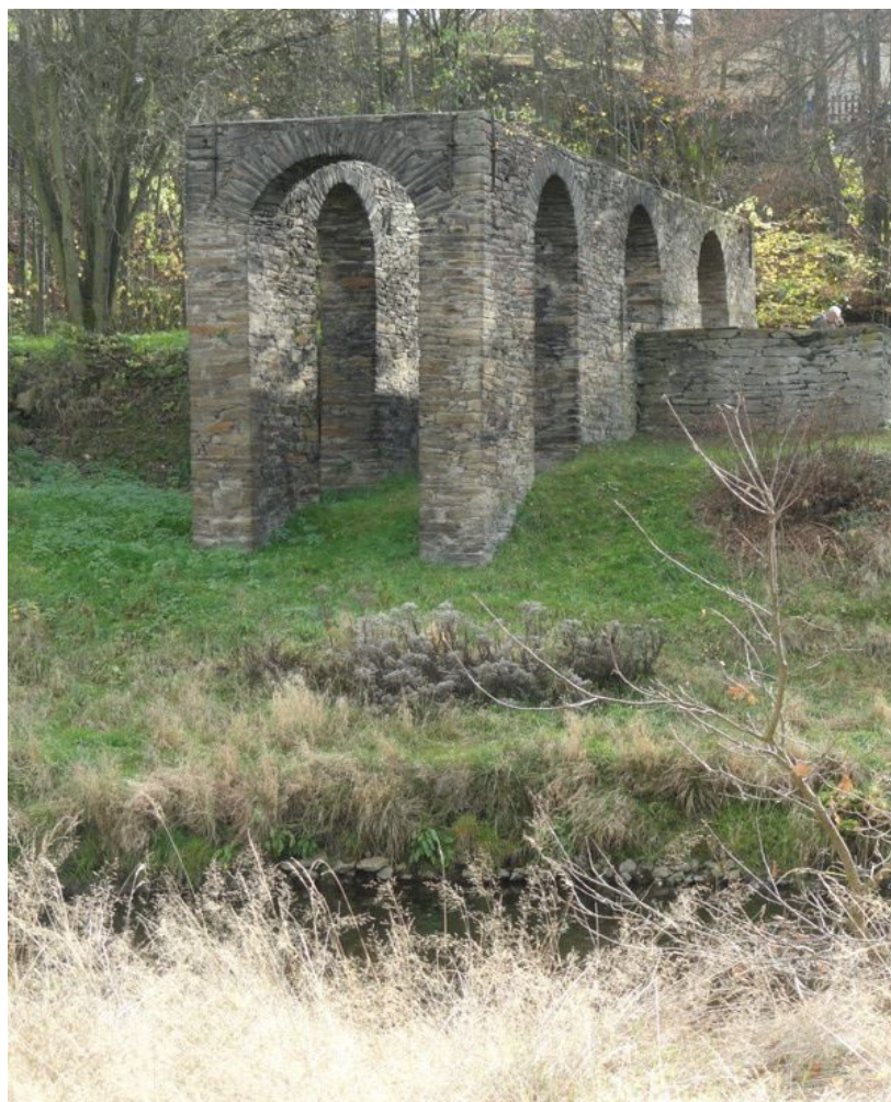
Early shiplift ruins of the ore transportation canal at the river Mulde, near Freiberg.
