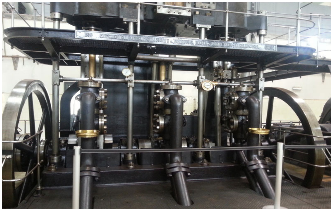
The steam pumping engines were manufactured in 1891 (the fourth one in 1904) in Karlín, today a district of Prague, by Breitfeld - Danek and Company (CKD). Pressure in the hydraulic system could reach 54 bar. Three of them were electrified in the 1930s and one was left intact.
