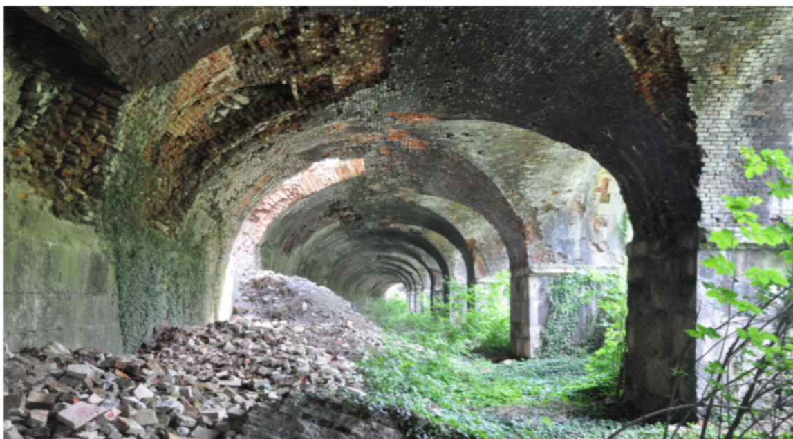
Inside the gallery: stones have fallen, bricks of the vault are flaking and sections of the gallery even broke down.
