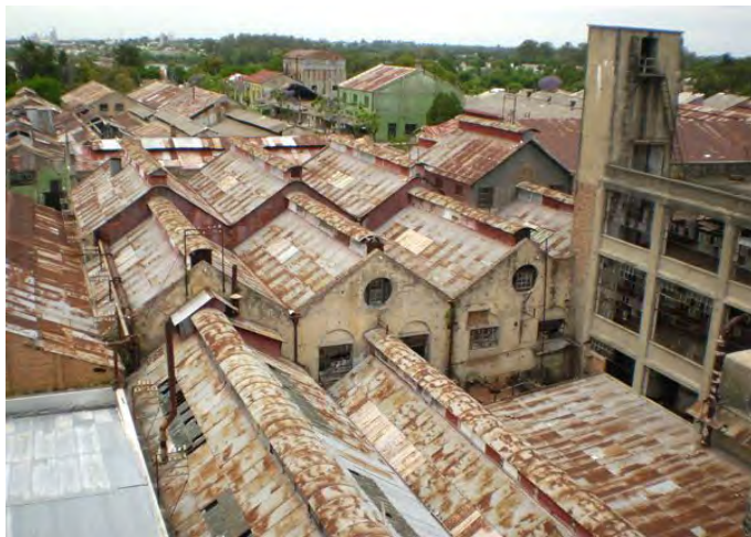
The rusting meat processing sheds of the Anglo factory, ©Ricardo Cordero
