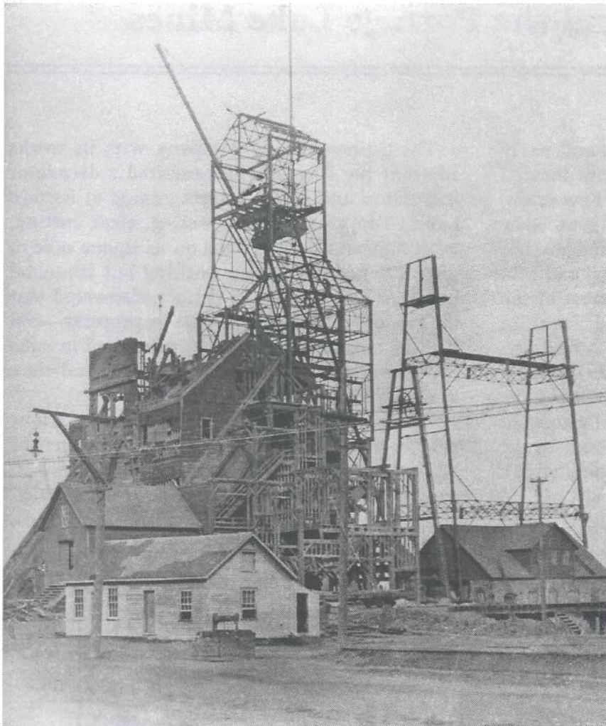
Quincy's steel-frame No. 2 shaft-rockhouse, shown under construction in 1908. (Historic American Engineering Record)
