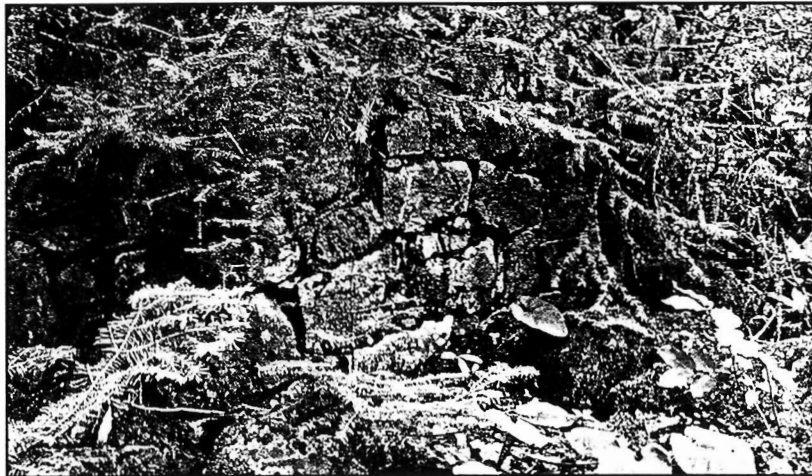
The stamp mill foundations of the Siskowit Mine as they now appear.
