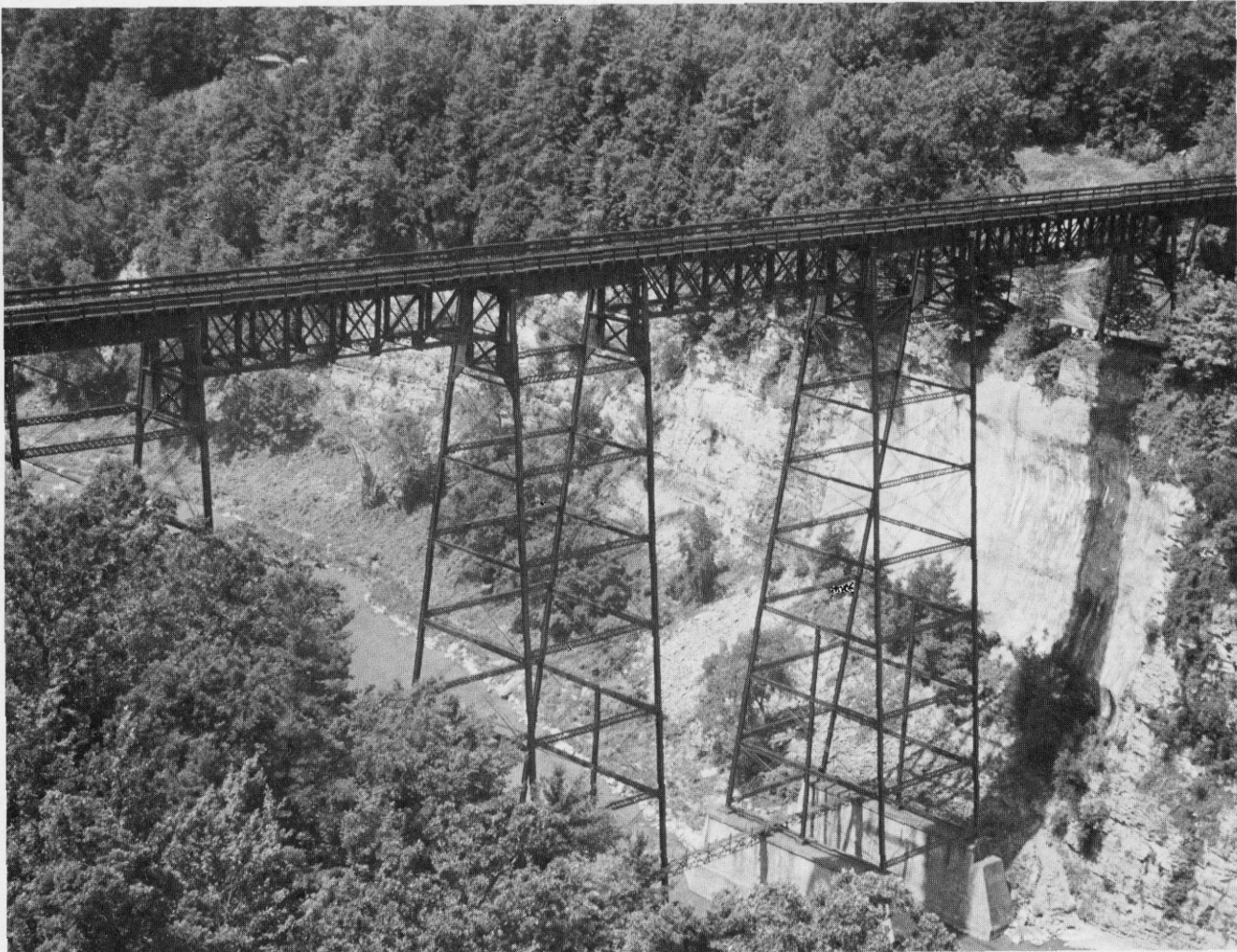
Portage Viaduct (1903), Erie Railroad. Jack E. Boucher for the Historic American Engineering Record, 1971
