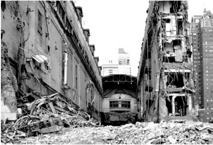
Waterside No. 2 being demolished. First view looks down what was once the turbine hall.
