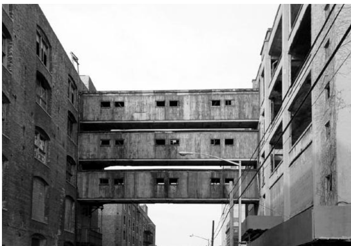
Bridges over West Street shown in March 2006 are now gone, pulled down after the fire due to instability of the rope factory structures they once connected.
