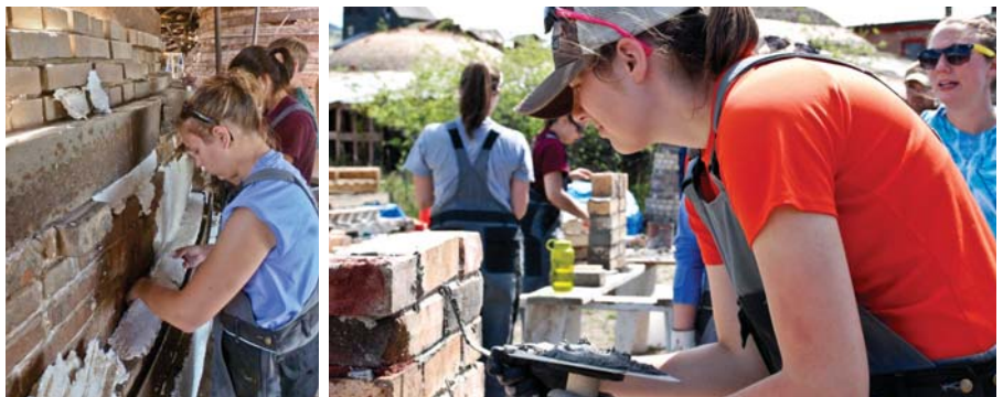
Far right: First laying a test wall with reclaimed brick. Christine Beckman then experiments with various repointing techniques on the same test wall. Immediate right: After drying for twenty-four hours, Jessica Focht and others remove a paper-based poultice mixed with detergent from the elevation of Kiln No.7.
