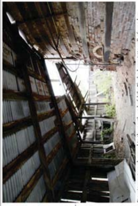
Framing system observed in the north end of kiln #7, abut consisting all of wooden members. The north framed opening in view (in background to the right).
