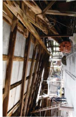
Condition of metal sheathing at the roof ridge between kiln #7 and #8. The left side of the ridge consists of corrugated metal sheets, while the right side of the ridge consists of standing seam panels.
