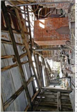
In the foreground, the stack exhaust fan installed in 1955 pierces the corrugated metal roof. Part of the corrugated metal roof is lifted to take account a raised ramp found below.
