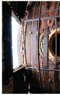
Framing system in the main span roof of kiln #7. After firing, the kiln doorways are opened releasing heat and water vapor. The framed opening allows the heat and water vapor to escape through the kiln shed.
