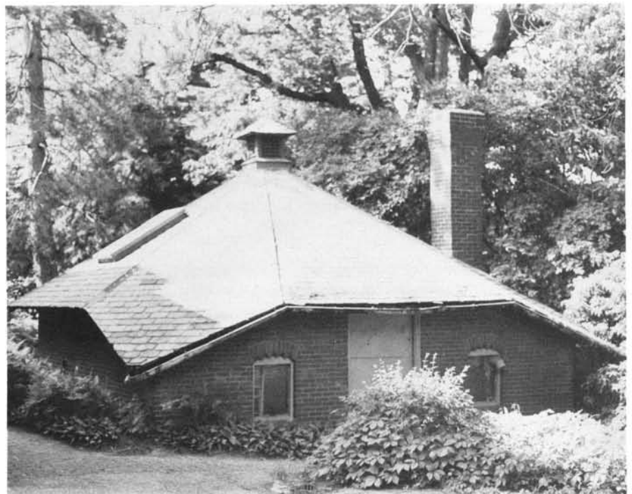
Figure 2. The gasholder house built c1855 by Samuel Cabot in Brookline, Massachusetts. Photographed in 1983 by the Brookline Historical Commission.
