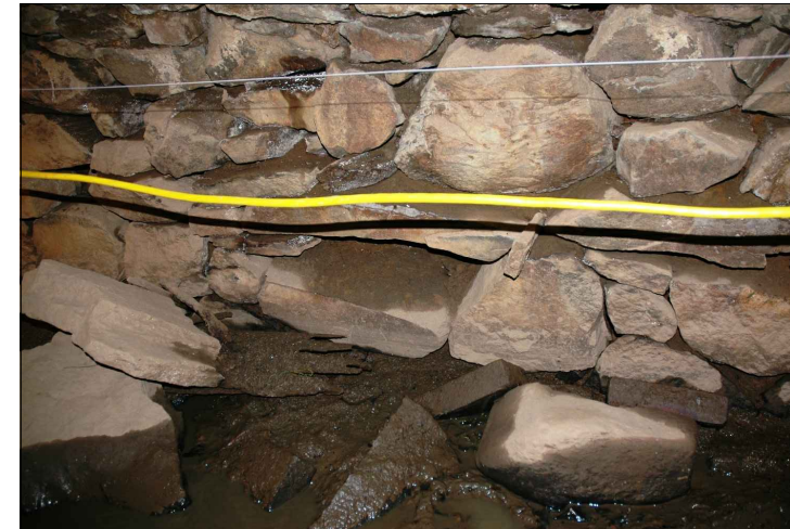
#47 STA 112 SOUTH: MANY STONES FELL OUT AT BASE OF WALL
