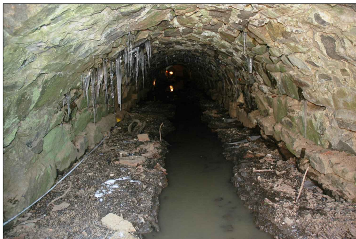
#102 STA 210 (LOOKING WEST): LICHEN ALONG WALLS, ICICLES FROM WATER INFILTRATION, CHANNEL ALONG TAILRACE BASE
