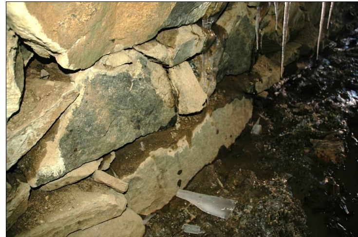
#96 STA 200 NORTH: STONES ARE DRY LAID, VOIDS BETWEEN STONES
