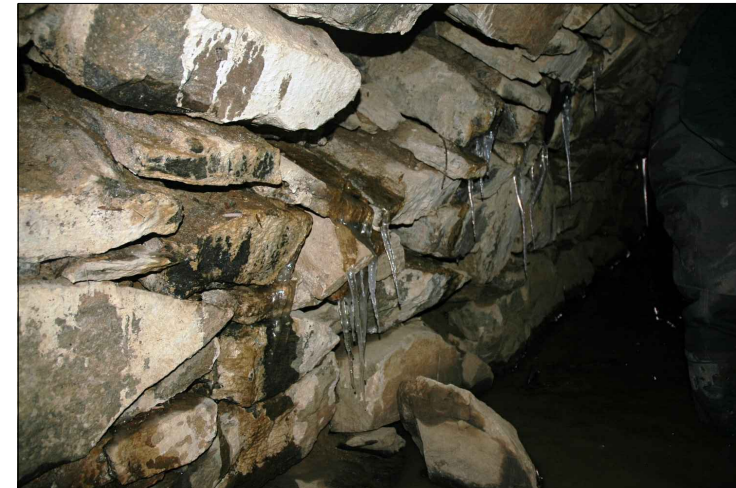
#73 STA 153 NORTH: STONE COLLAPSE, ~24"
