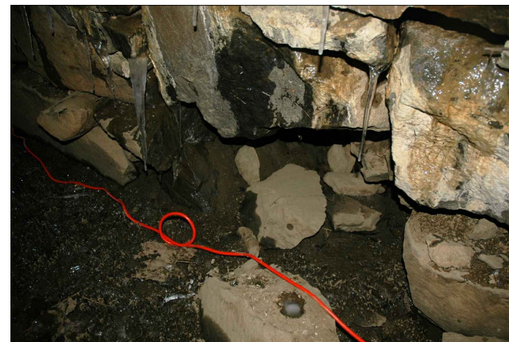
#77 STA 160 SOUTH: STONE COLLAPSE, ~30"
