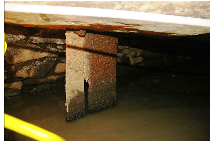
#129 STA 16 SOUTH (ENTRANCE TO SAWMILL TAILRACE): STEEL SUPPORT PLATE IS SEVERELY CORRODED
