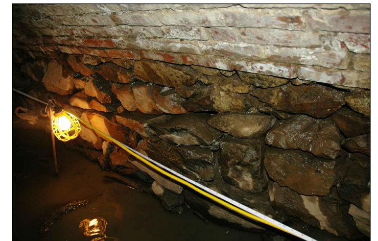
#11 STA 94 SOUTH: STONES ARE BULGED
