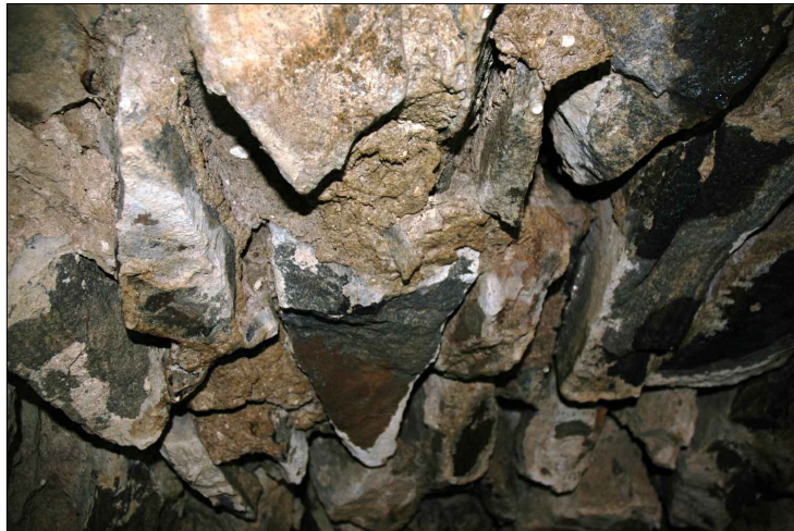
#71 STA 150: OVERHEAD STONE IS DRY LAID
