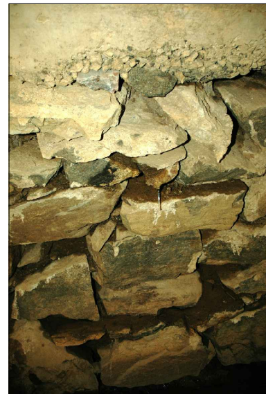
#62 STA 140 NORTH: LOOSE STONE
