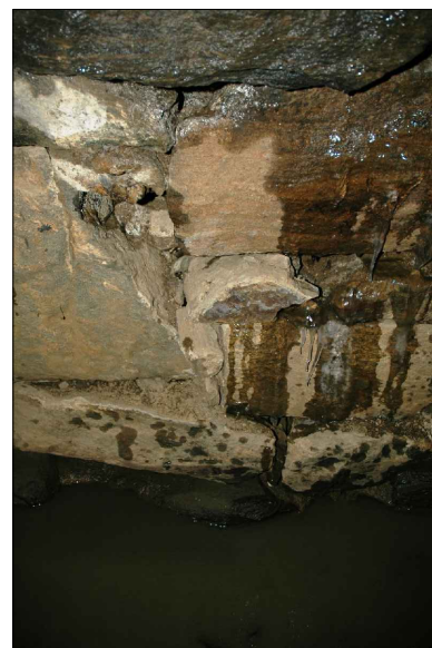
#83 STA 180 SOUTH: STONE LOSS AT BASE, ~14"
