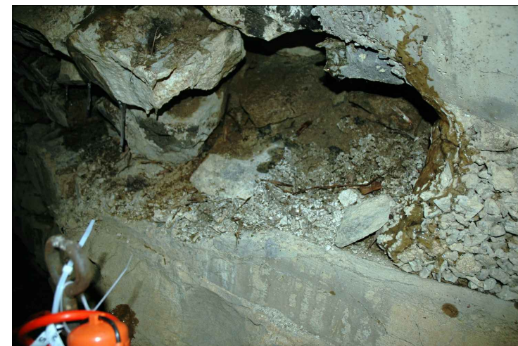
#72 STA 151 SOUTH: STONE COLLAPSE, ~16"
