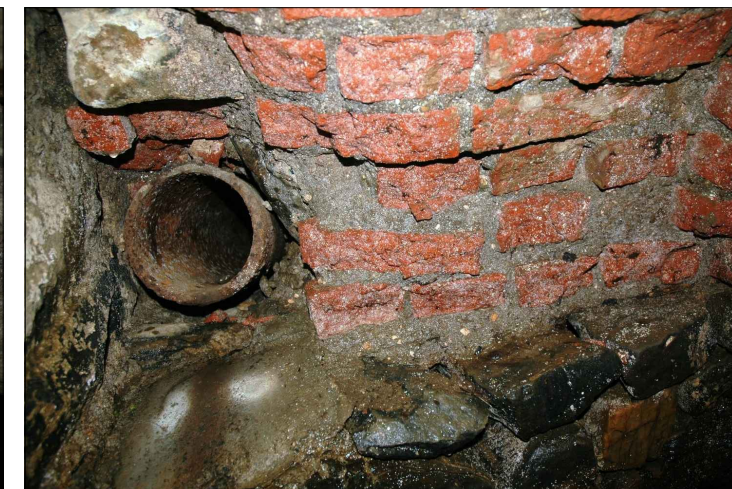
#121 STA 5'-5" NORTH ELEVATION: TERRA COTTA DOWNSPOUT
