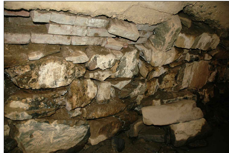
#59 STA 130 NORTH: LOOSE STONES, BRICKS FALLING OUT FROM WALL
