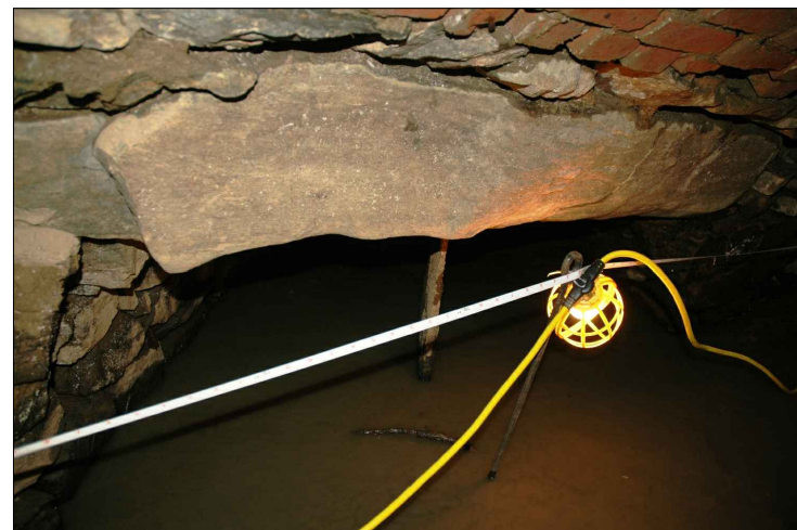
#133 STA 19'-5" SOUTH": EAST END OF STONE LINTEL IS UNSUPPORTED
