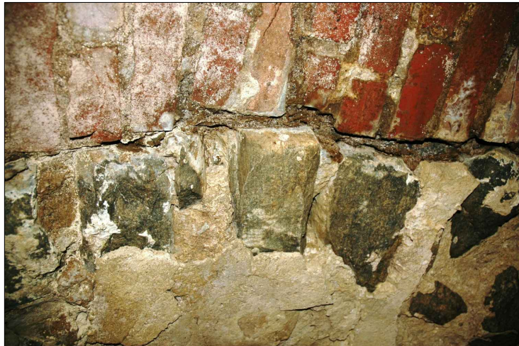
#19 STA 71'-5": TRANSITION BETWEEN BRICK & STONE IS NOT KEYED INTO EACH OTHER
