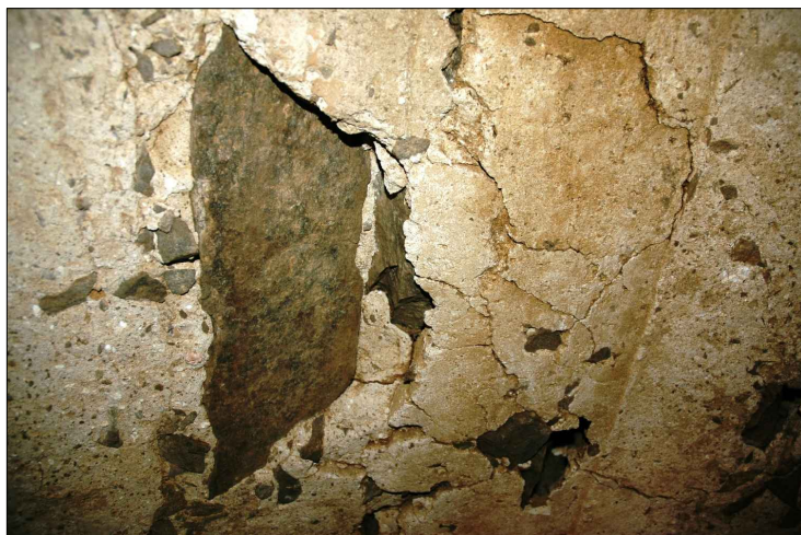
#24 STA 60: OVERHEAD PARGING IS CRACKED
