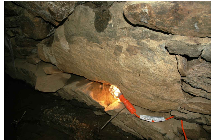
#82 STA 170 SOUTH: LOOSE STONES AND VOIDS
