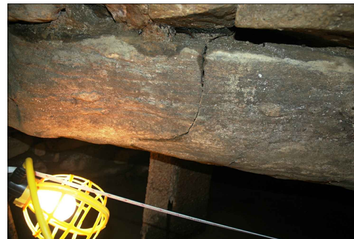
#126 STA 16 SOUTH (ENTRANCE TO SAWMILL TAILRACE): VERTICAL CRACK AT MIDPOINT OF STONE LINTEL
