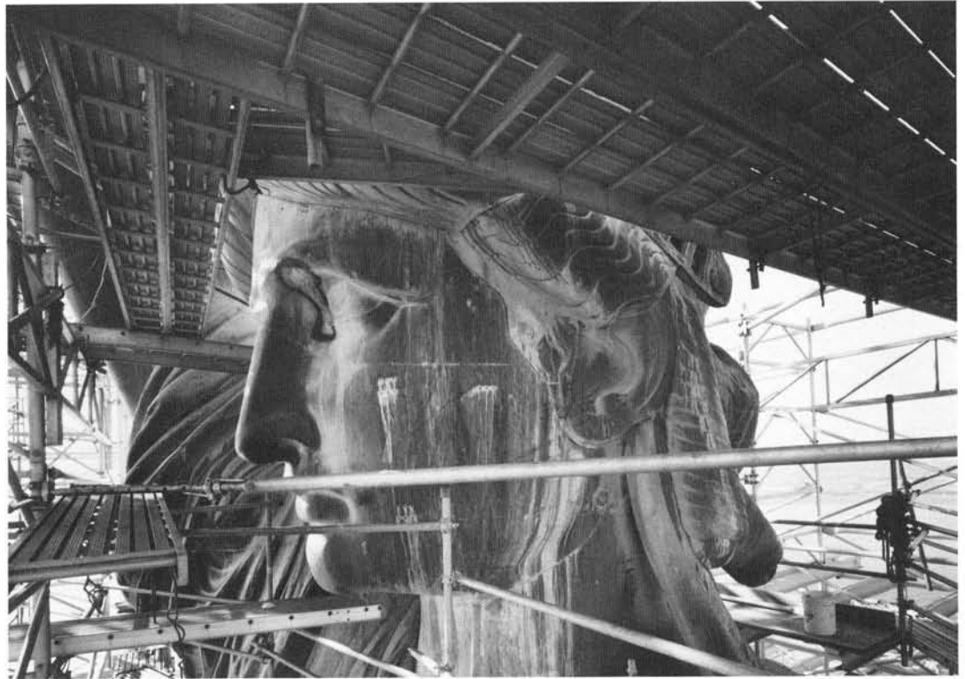
Liberty's magnificent head. The dark area at the eye marks a graft of new copper skin. The lobe of the nose also has been repaired. Streaks on the face and neck were caused by a bicarbonate-of-soda solution, used to remove coatings on the interior surface, which oozed through joints between copper plates and through the holes for rivets connecting the skin with iron support straps on the inside. Jet Lowe photograph for HAER (12-85).
