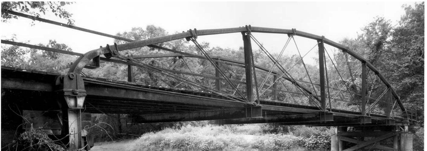
Figure 5: One of five extant Horton bowstring trusses in the VanLoon Wildlife Area north of Lacrosse, WI. Source: HAER WI-22B-2.
