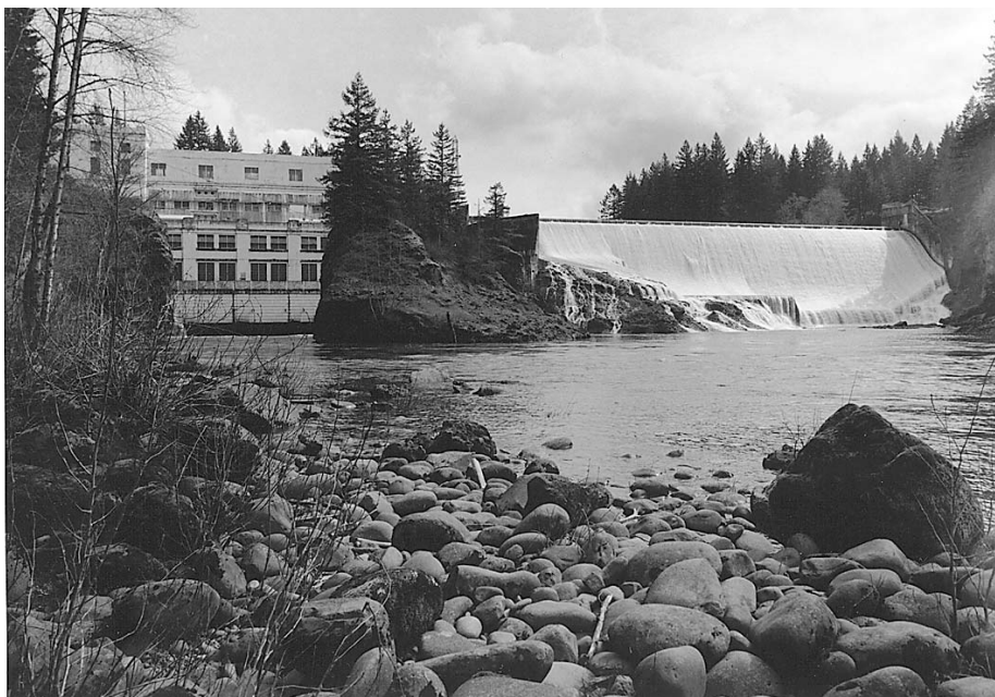
River Mill hydroelectric plant and dam, Estacada, OR.
