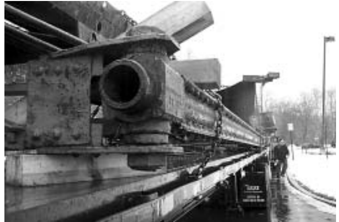
Doty Road Bridge’s Phoenix Column upper chord aboard a flat bed trailer on its way back home to Phoenixville, PA.
