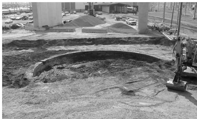
Portion of retaining wall for turntable pit, New Haven rail yard roundhouse, 1870. Piers in background are for the Church St. overpass.
