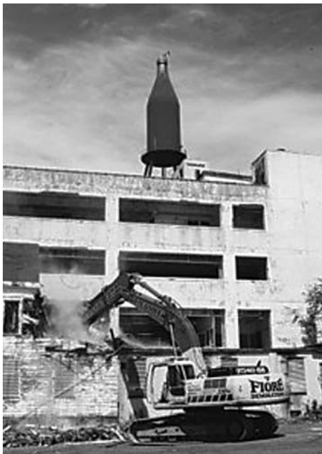
Newark, NJ, wants to save the famous beverage bottle from atop Pabst's main building but has begun demolition of the brewery complex.
