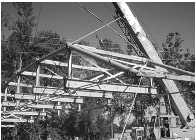
A crane prepares to set the restored Aldrich Change Bridge on its new abutments.
