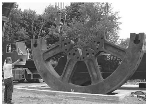
One of the 60,000-lb. flywheel halves being lowered into the flywheel pit by both Grove cranes.
