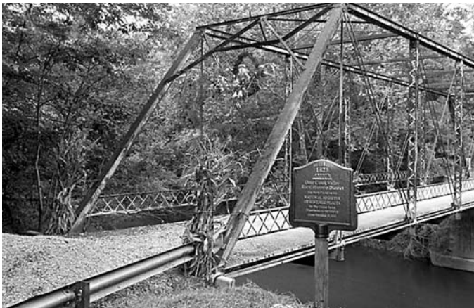
Wilson Bridge (1898) has been at the center of a test case on Indiana's historic bridges. HAER Collection, Library of Congress.
