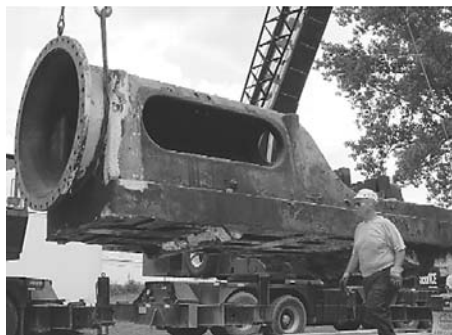
A Grim's Crane Service employee watches as the lowboy truck is pulled out and the low pressure bedplate is lowered into position.
