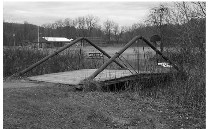
The Cummington (MA) Ball Pipe-Truss Bridge has been rehabilitated and preserved as a pedestrian bridge on a trail behind the local elementary school.
