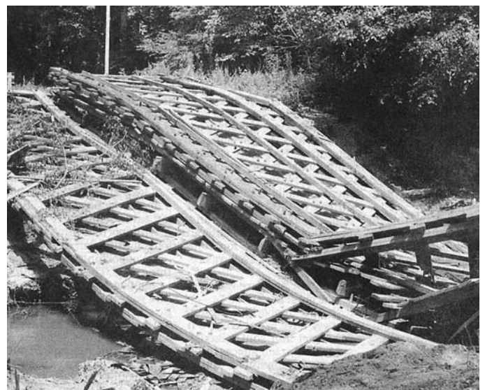
The collapsed Town-lattice trusses of the Salem-Shotwell Bridge, June 2005. The trusses have since been salvaged and will be repaired and re-erected at a new location.
