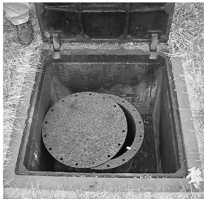
Pump-out port for separator tank.
