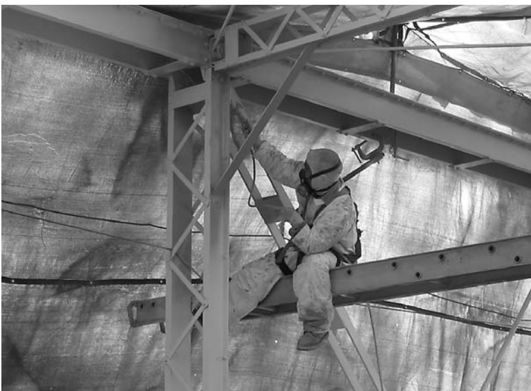
Inside the cocooned bridge, workers removed lead-based paint and applied new paint.
