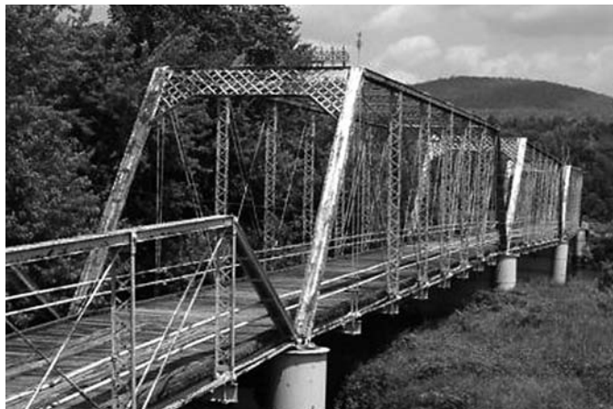
Meadow Bridge in Shelburne, NH, is one of only two bridges thus far to receive a Save America’s Treasures Grant.
