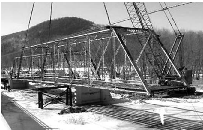
One of the spans of the Meadow Bridge being lifted by a crane in Feb. 2004.
