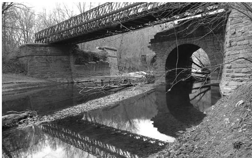
The remaining stone arch and abutments of the Catoctin Creek Aqueduct. The center span collapsed in 1973 to be replaced by the Bailey truss bridge.
