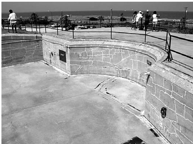
Emplacement for 12-in. gun paved over for use as an observation platform.
