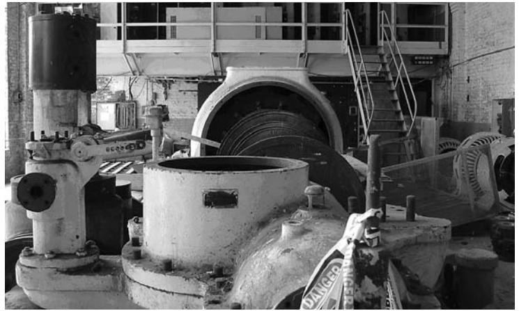
Turbine Room, 2006. The mezzanine was added at a later date for updated electrical controls; turbine in foreground.
