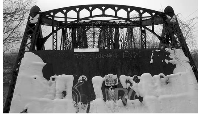
Portal of the Schell Bridge. The steel plates were welded to the bridge portals in 1987 but some of the Gothic Revival-details can still be seen.
