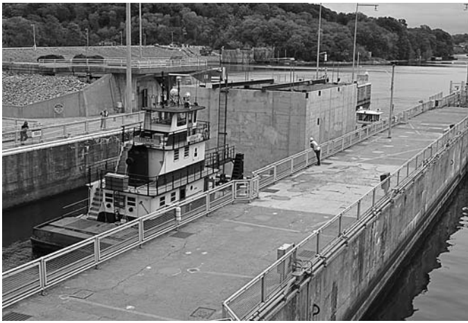
The Chickamauga Dam navigation lock. The tugs are directing a precast concrete foundation block through the lock. The block will be sunk to the riverbed and form part of the foundation for a longer and wider lock that will replace this one.
