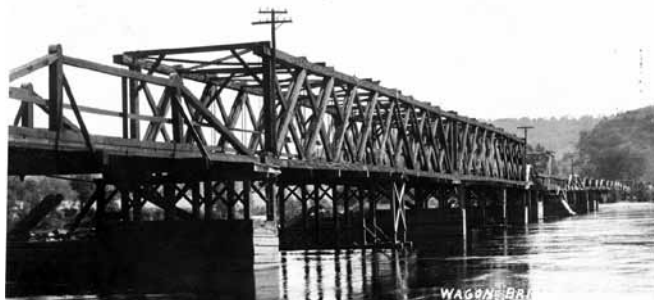
Wagon bridge, a Howe with vertical end posts. Prairie Du Sac, Wis.
