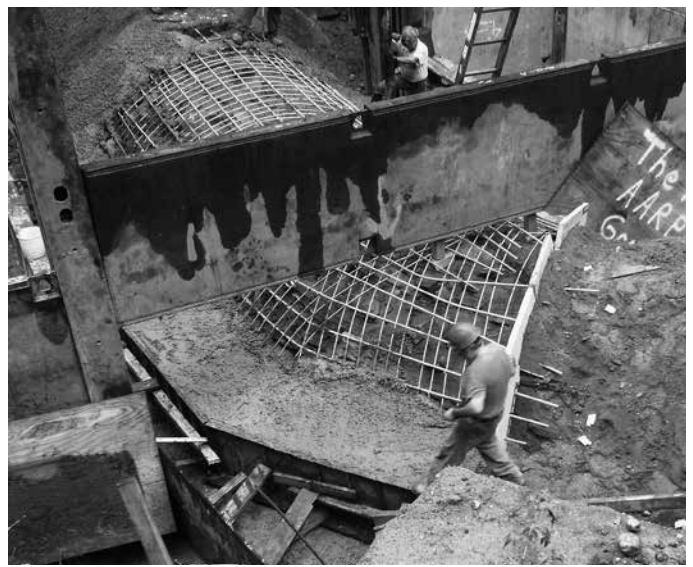
Reinforcing bars being placed to strengthen the tunnel arch. Note the bend in the tunnel.
