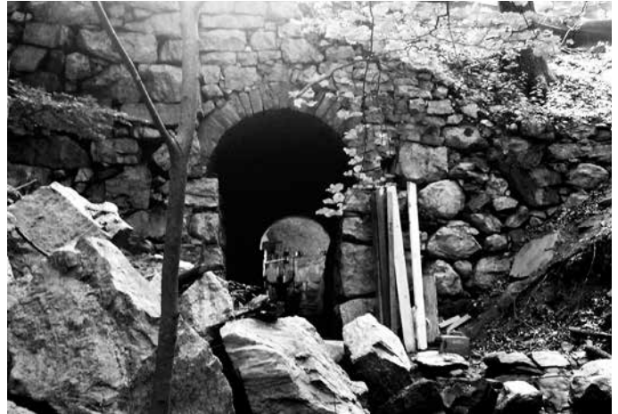
Bracing the interior of the Davis Brook tunnel for repairs in a view from the western portal.
