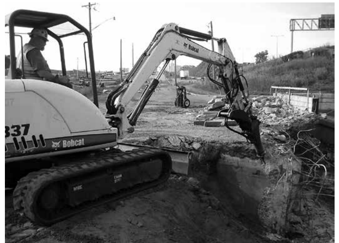
Careful demolition of the bridge revealed the reinforcement, facilitating its documentation in selected areas: a full-depth opening was made near the center of the bridge span (top); the slab edge was deconstructed at the connection of the deck to the abutment (center); and the abutment wall was chipped away.
