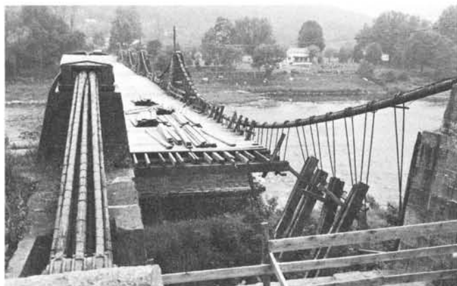
The damaged aqueduct—looking toward Penna. from the N.Y. abutment. On left are the cable strands, attached to the links of the anchor chains (bottom) and covering at the first tower saddle, just beyond which they are bundled into the characteristic cylindrical form as seen on the right.
